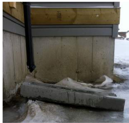
Ensure exterior discharge for sump pump is clear of ice or debris and drains onto a positive slope away from the house.
