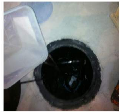
To test sump pump, fill hole with water (by bucket or hose) to about 1 foot above bottom. The round float will rise and when it hits a certain threshold the pump will activate.
