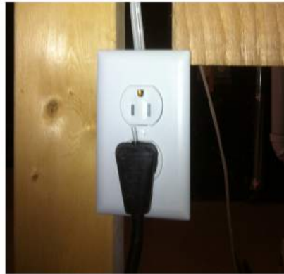
Ensure sump pump is plugged in to the inverted outlet and that outlet has power.
