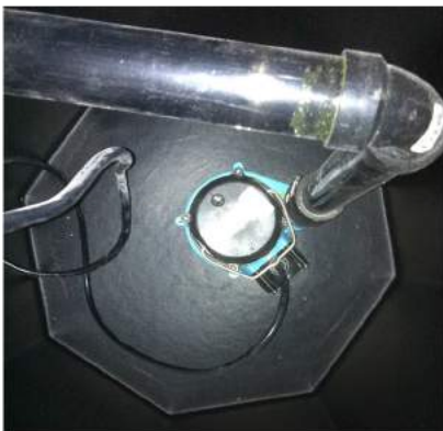
Inspect components to ensure proper connections. Note: it is not uncommon for sumps to have sitting water in the base.
